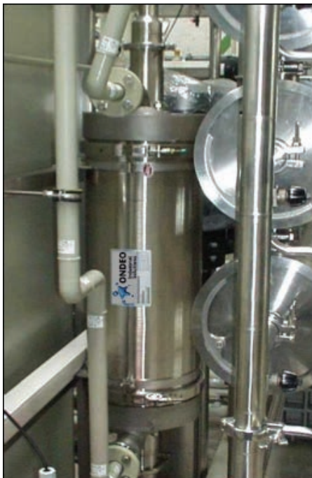
Contactors in an 8 m 3 /h ROCEDIS plant
