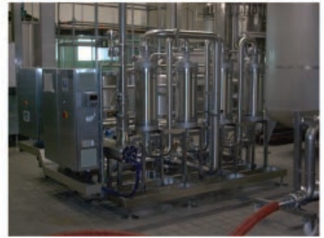
Figure 5: The Water Deaeration System DGS 400 has been in operation since October 2003 and has not required problem solving or maintenance.
