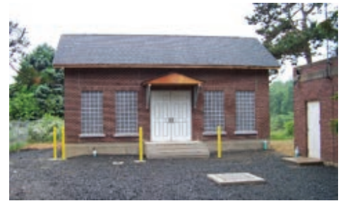
A building erected around the Liqui-Cel membrane contactor system. This installation is in a residential area, so it was important to conceal equipment in an aesthetically pleasing manner.
