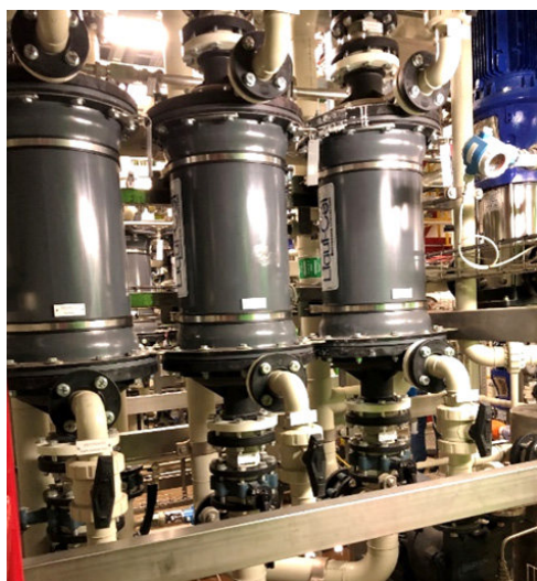
Figure 3: Three 3M Liqui-Cel EXF-14×28 Series Membrane Contactors
